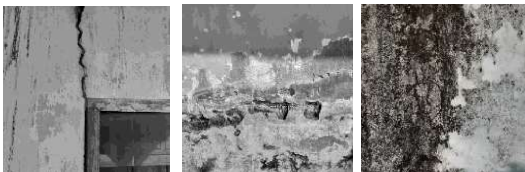
Figure 1. Various surface damages of concretes as a result of its exposure to atmospheric conditions.
